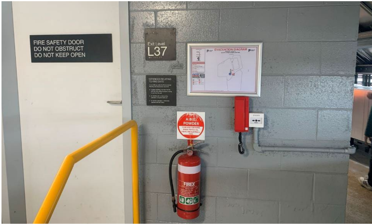
Evacuation diagram displayed in the plant room, with a fire extinguisher mounted on wall.
