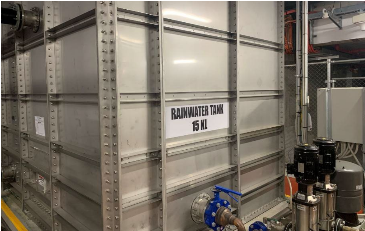
15 kL rainwater tank installed for the collection and storage of rainwater. The water is reused on-site for landscaping irrigation purposes, supporting sustainable water management practices.
