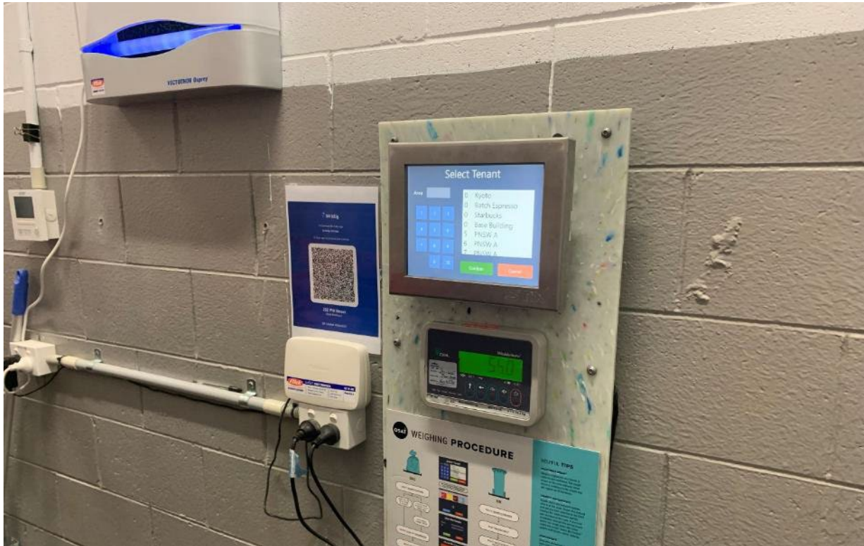
Weighing machine installed in the waste collection room to measure bins and record data on waste disposal.
