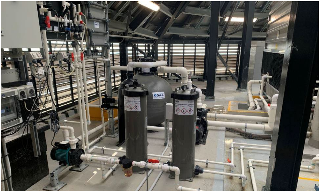
Chemical dosing system and associated filtration units within the plant room.
