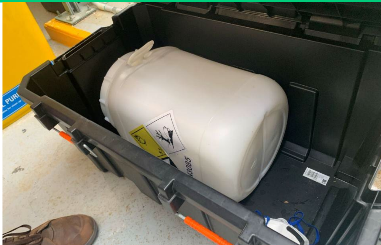
Chemicals noted to be bundled in plant room.
